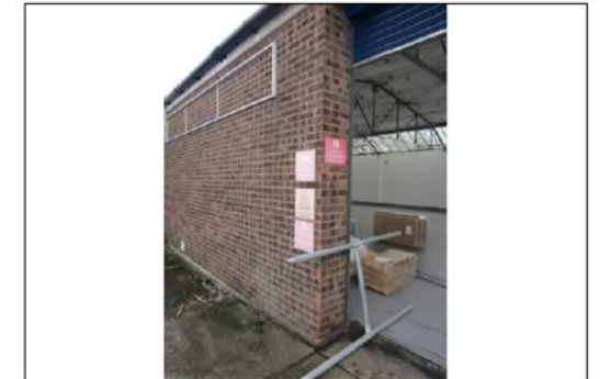
22. View showing further impact damage to left-hand side of roller-shutter.
