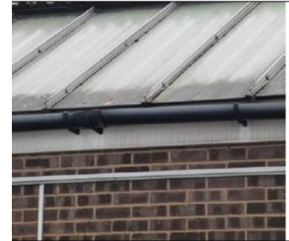
20. Showing PVC fascia. Heavily begrimed and stained.
